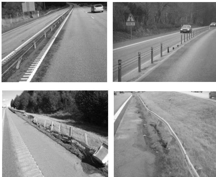
Figure 5.12 Damaged road barriers due to vehicle collision
