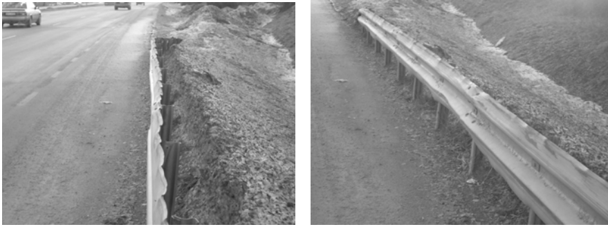
Figure 5.13 Damaged w-beam barriers due to impact by snow removal equipment
