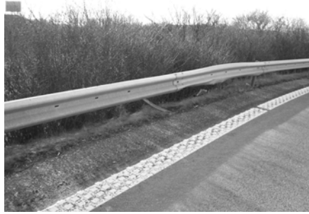
Figure 5.4 A damaged w-beam barrier which still retains some degree of efficiency
