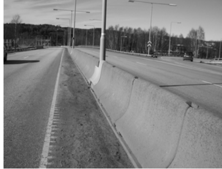
Figure 5.7 Safety shape barriers
