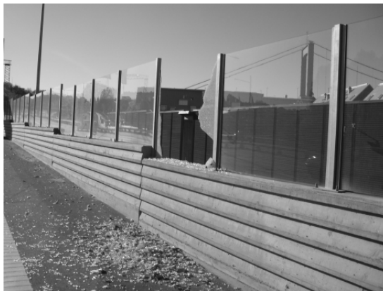
Figure 1.1 Damaged noise barrier along road E6.20 in the city of Gothenburg in Sweden
